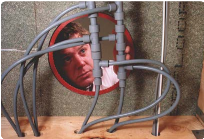
Plumbing (hot and cold water)
